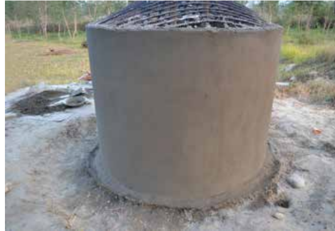
Figure 39: shows the tank with the completed outside layer of plaster. Finished exterior coat
