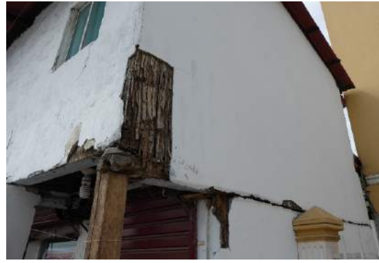
Figure 41: Spalling of render after earthquake, revealing rotten bamboo esterilla below, Ecuador (Kaminski, 2016)
