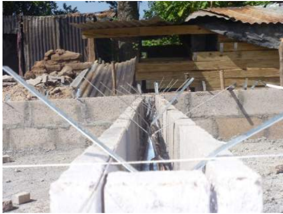
Figure 64: Photo of sole plate fixed to upstand with cast-in off-the-shelf steel straps, before casting straps into reinforced blockwork
