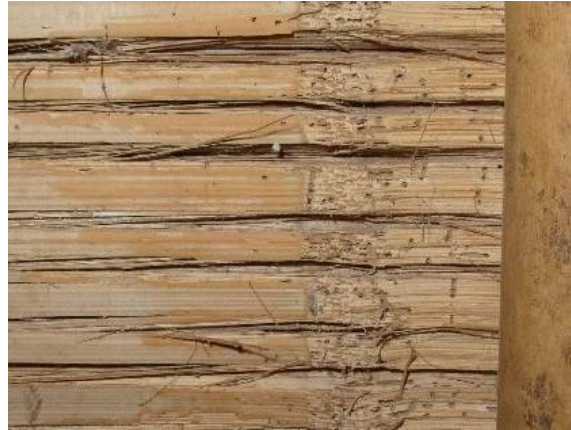
Figure 31: Beetle damage in bamboo, Colombia – exit holes are clearly visible (Kaminski, 2016)
