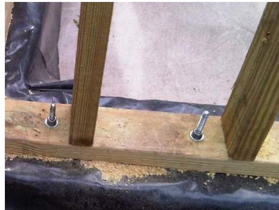
Figure 61: Detail of sole plate fixed to upstand with bolts Figure 62: Photo of sole plate fixed to upstand with bolts
