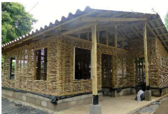
Figure 24: Cane and timber housing, El Salvador – before application of render. Note the large overhangs on all sides and the elevated frame on a damp-proof membrane (Kaminski, 2016)
