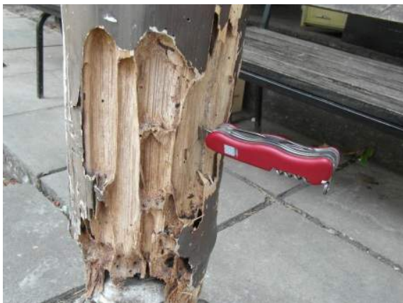
Figure 34: Severe termite damage in bamboo, Costa Rica. Note how the outer painted silica shell of the bamboo is still intact in some areas and hence appears in good condition (Kaminski, 2016)
