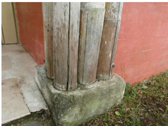
Figure 38: Fungal damage, splitting and bleaching of boron-treated bamboo exposed to the sun and rain after around 10 years, Colombia (Kaminski, 2016)
