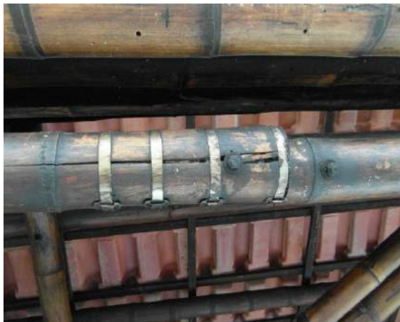
Figure 73: Steel pipe ties used to strengthen bamboo after it had split, Colombia (Kaminski, 2016)
