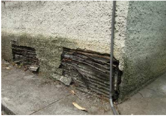
Figure 40: 100% section loss of cane to the base of walls, Costa Rica. Note the mould visible at the base of the walls due to splashback from the roof. The cement and paint is clearly not sufficient protection under driving rain (Kaminski, 2016)
