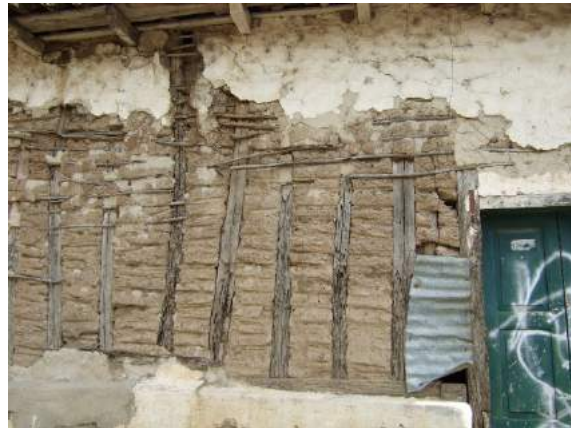
Figure 33: Severe termite damage to timber and cane in traditional bahareque, El Salvador (Kaminski, 2016)
