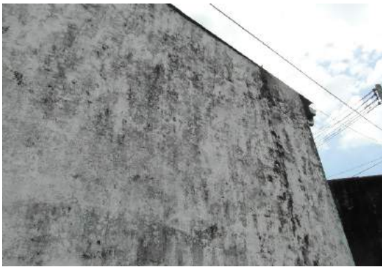
Figure 42: Engineered bahareque house in Colombia with no roof overhang – the mould on the wall is clearly visible (Kaminski, 2016)
