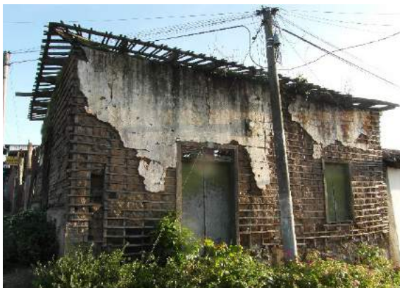
Figure 3: Traditional bahareque housing in Berlín, El Salvador. The outer render has spalled off (Kaminski, 2016)
