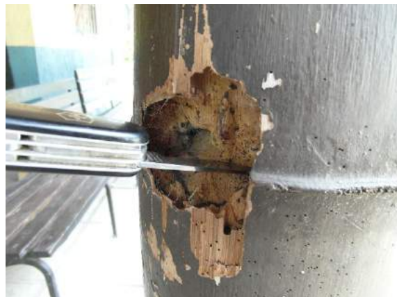
Figure 35: Severe termite damage in bamboo, Costa Rica. The small round black drywood termite droppings are just visible (Kaminski, 2016)
