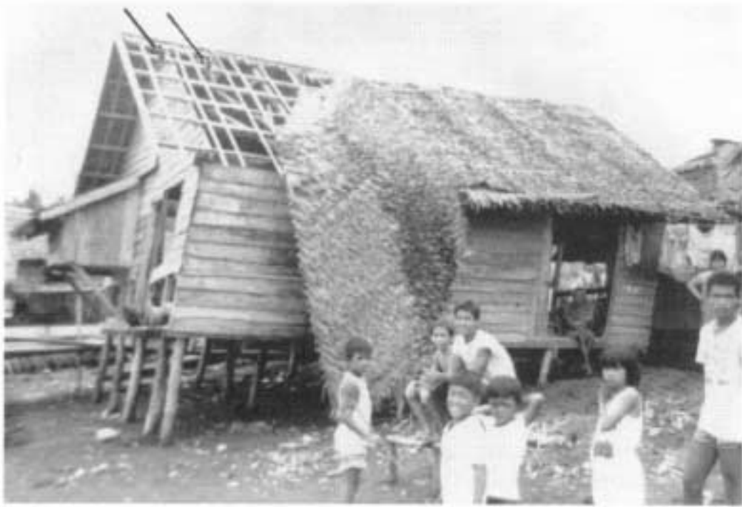
Fig. 4. Failure of a roof in which nipa tiles were tied at only two points (position of missing bamboo splits arrowed).
