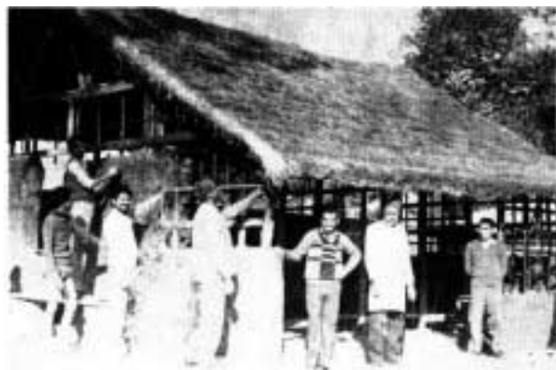
Fig. 2. Bamboo house showing roof covering (by thatches), bamboo truss and bamboo-reinforced mud wall (construction in progress).
