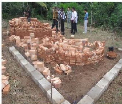
Plate 8: Perspective view showing the cement block wall and two brick kilns under construction
