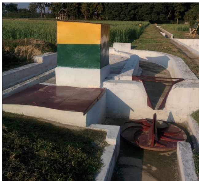
Fig. 3.8: H-flume installed at research farm of ICAR - IISWC, Dehradun (India)
