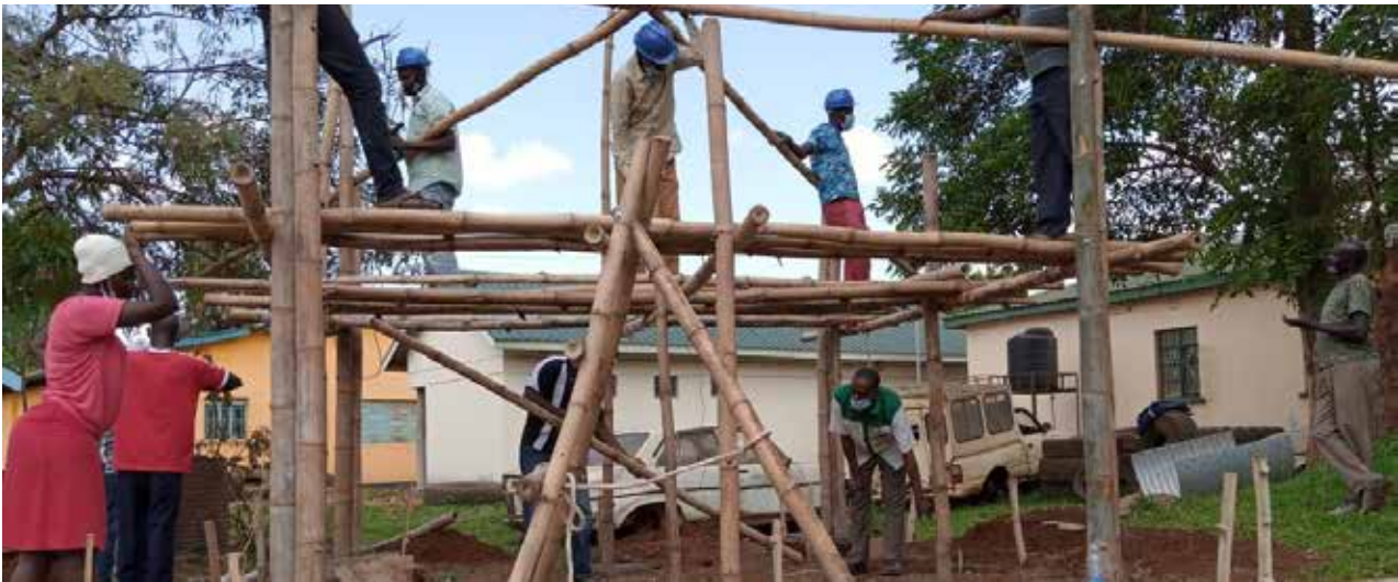
A gazebo being constructed in Busia county, Kenya, as part of the Dutch-Sino-East Africa Programme.
