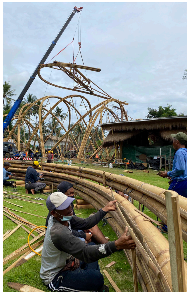
A crane lifts an arch into position for the Arc structure at Green School, Bali. Credit: Elora Hardy.
