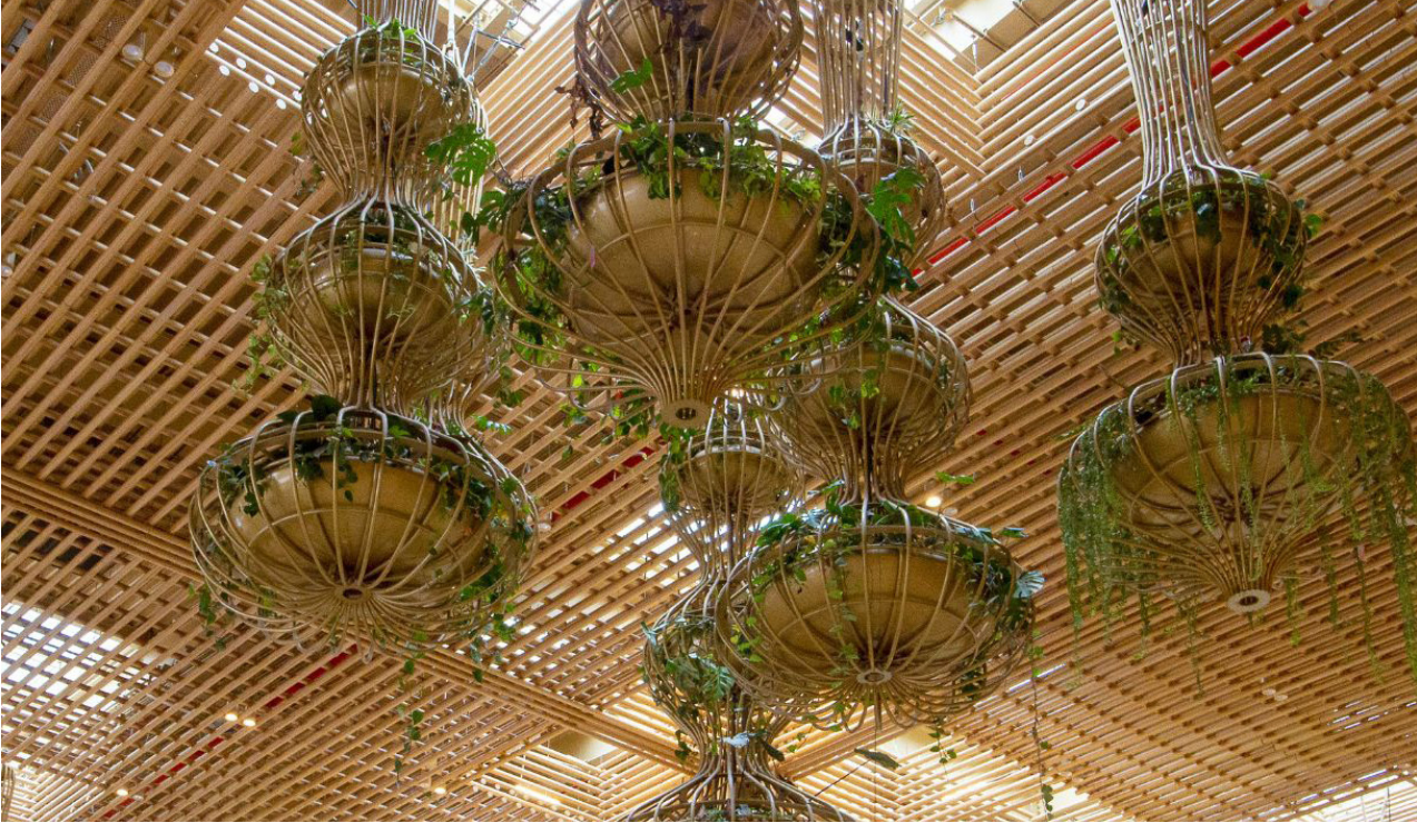
Engineered bamboo adorns the ceilings and walls of an airport terminal in India. Credit: MOSO International.
