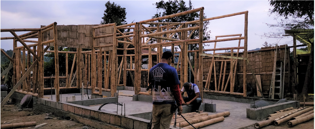
Bamboo construction experts are building new homes and new futures for rural Ecuadorians.
