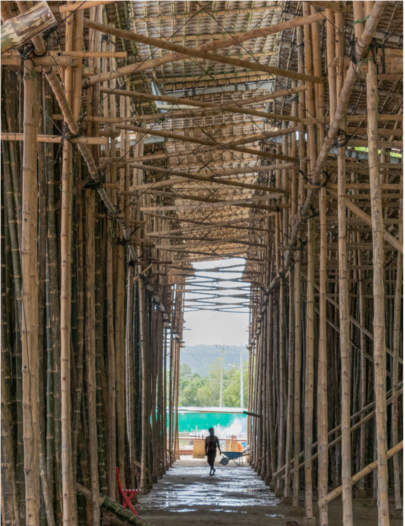
Bamboo treatment facility providing durable bamboo solutions to Rohingya refugees. Credit: Nate Webb/IOM
